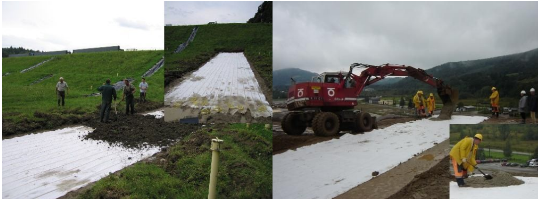
Figure 1. Installation of sensitive non-woven mats with standard silica fiber sensors in Solina (left) and in Swinna Poremba (right) – Poland.
