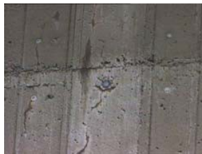
Figure 3. Picture of a defect captured with SCANSITES®.
