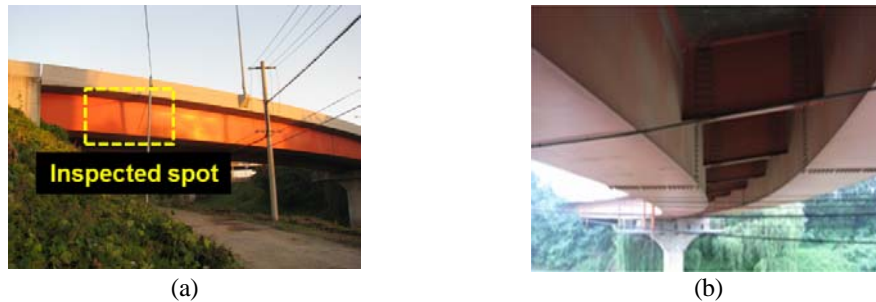
Figure 5. Ramp-G bridge in South Korea and the inspected spot. (a) Overview of the bridge and (b) bottom view of the bridge.
