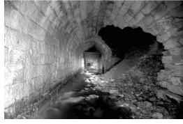
(a) Tunnel Collapse
