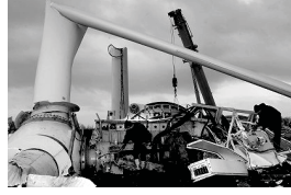
(b) Turbine Collapse
